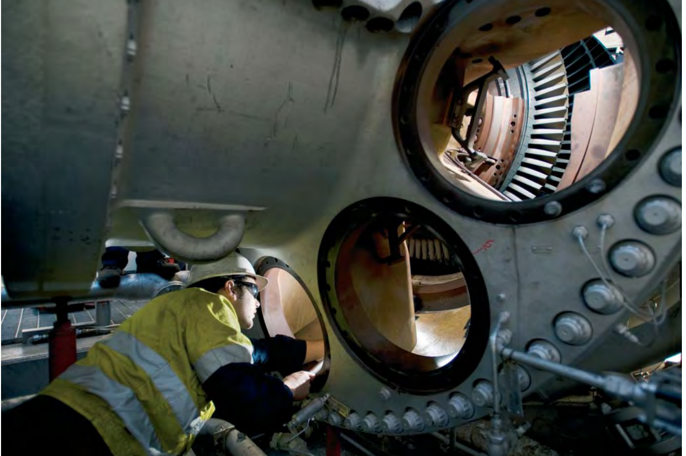
Inspection of the Mica Creek Power Station Unit A6 turbine during this year's planned overhaul
